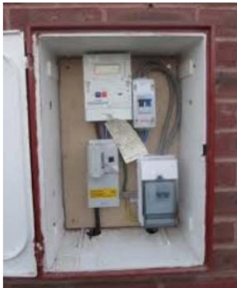
Figure 20. External electricity meter
