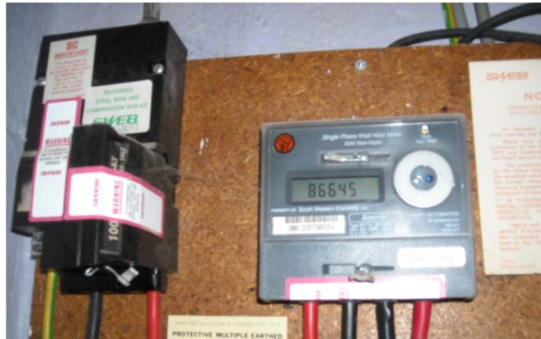
Figure 21. Internal electricity meter
