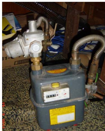
Figure 27. Internal gas meter
