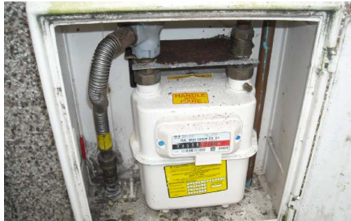
Figure 26. External gas meter
